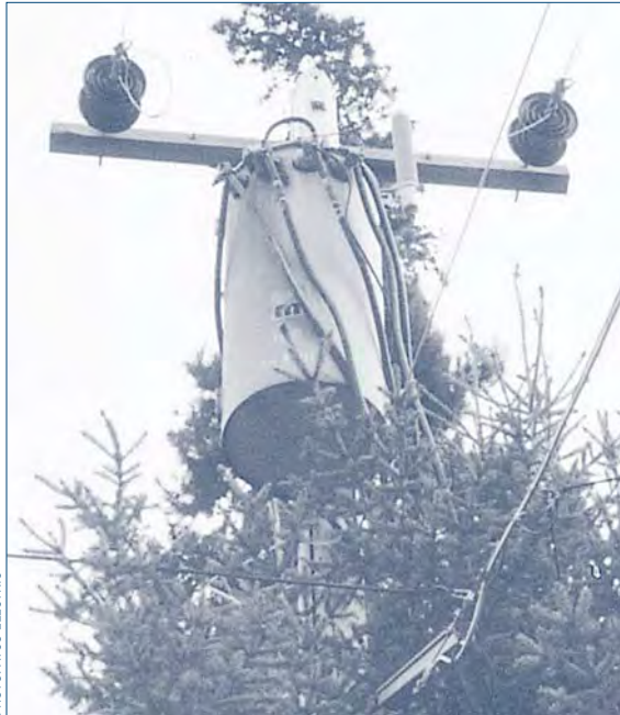
PHOTO: ATCO ELECTRIC
