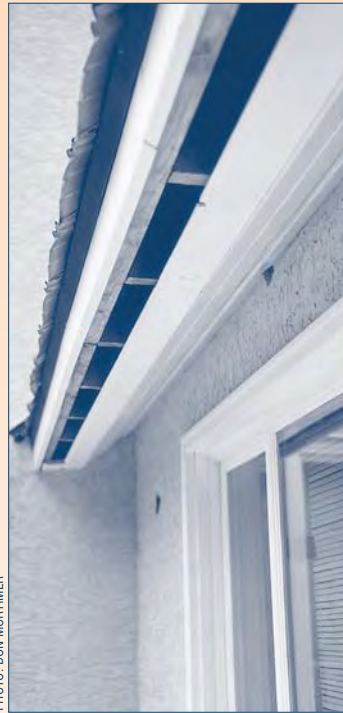
▲ Closed eaves, vents not screened with 3-millimetre mesh. (1 pt)
