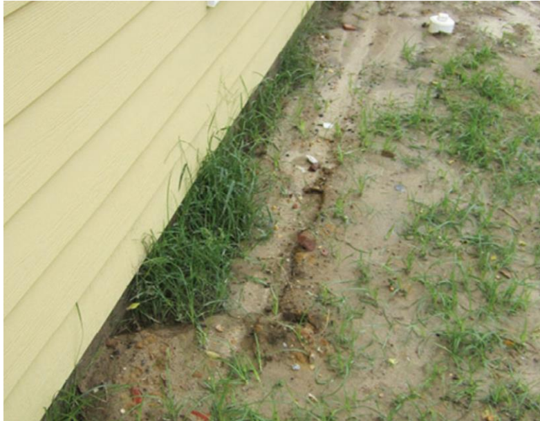
Figure 18 - Erosion and water damage as a result of roof runoff impacting the ground (image courtesy Building American Solution Centre)
