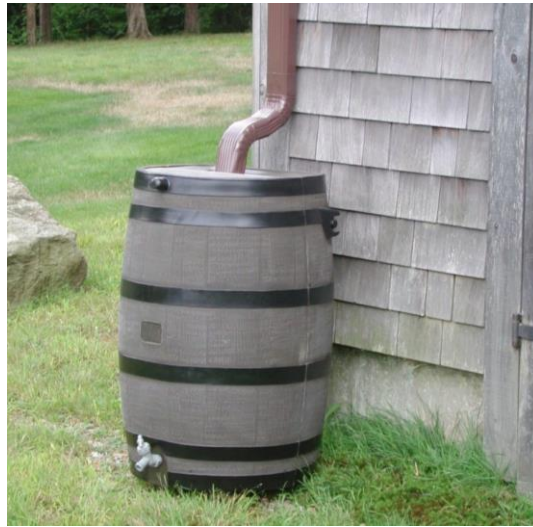
Figure 22 - Rain barrel at end of downspout to collect rain runoff from roof for use around property (image Pinterest)
