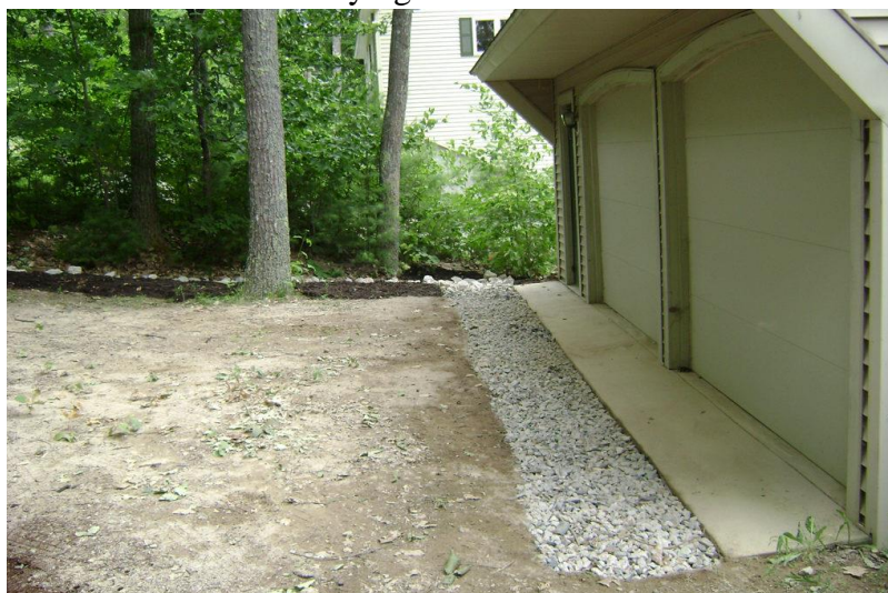
Figure 23 - Dripline-trench installed below edge of roof to prevent erosion as a result of roof runoff (image courtesy Acton Wakefield Watersheds Alliance)
